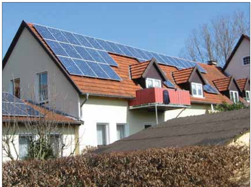
Photo 1. Residential PV installation
