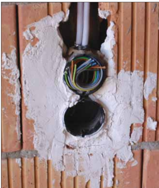
Photo 4. Fine stranded cables used for residential wiring
